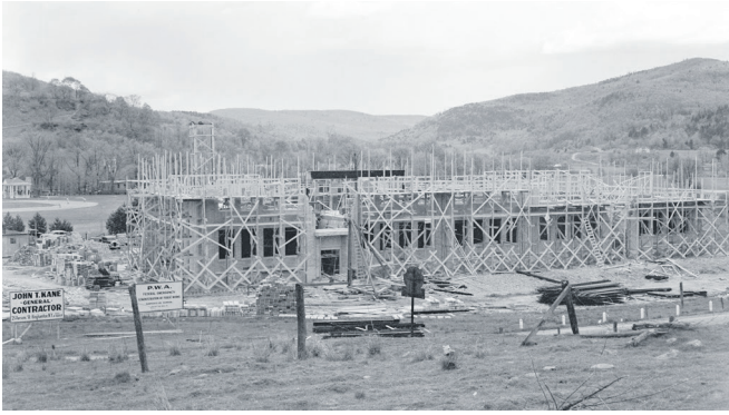
Photo Contributed by DCHA, Bob Wyer Collection Construction of Downsville Central School, May 1939.
